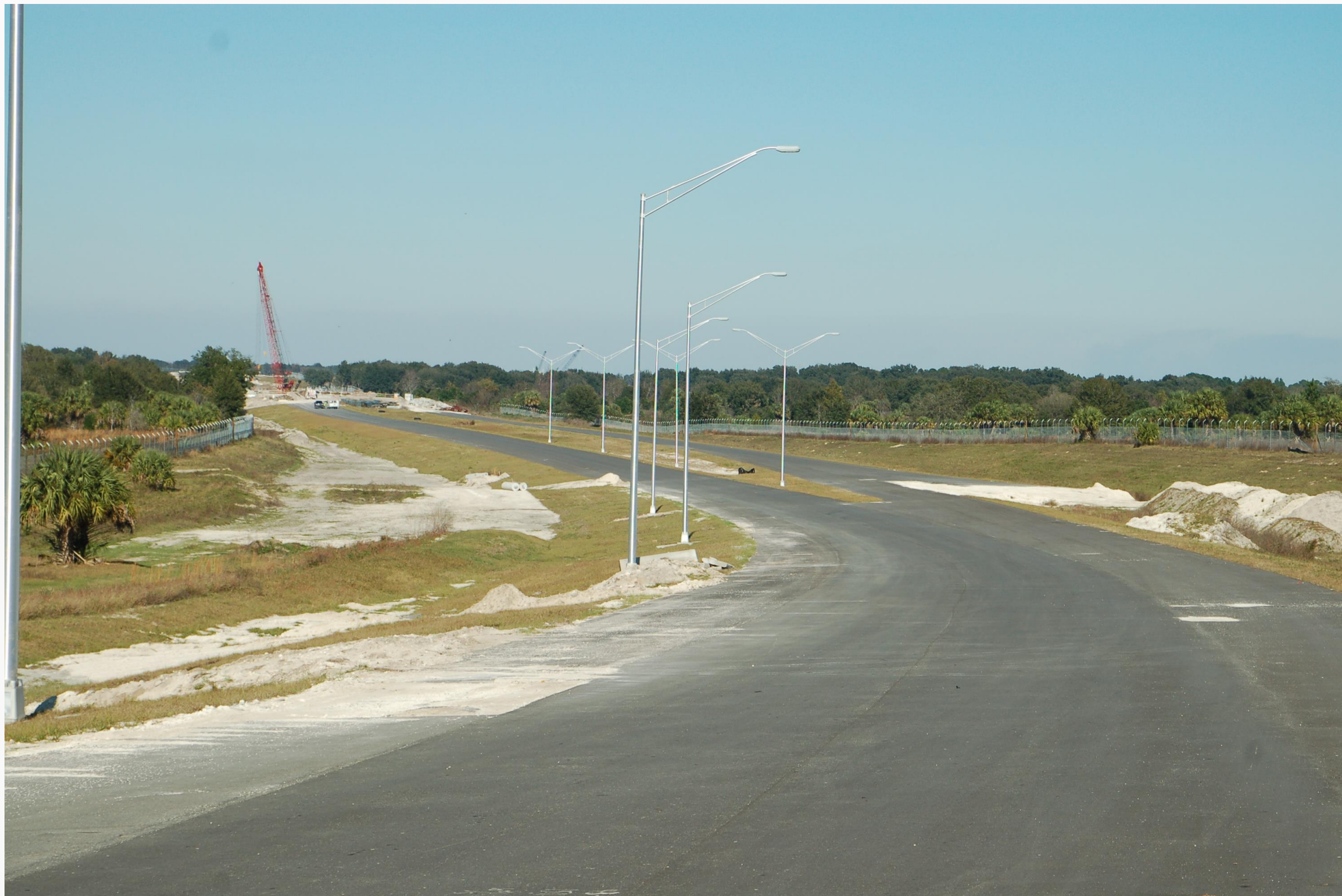
Pavement, street lights and wildlife fencing on Section 4A near CR 435 (Mt Plymouth Road)
