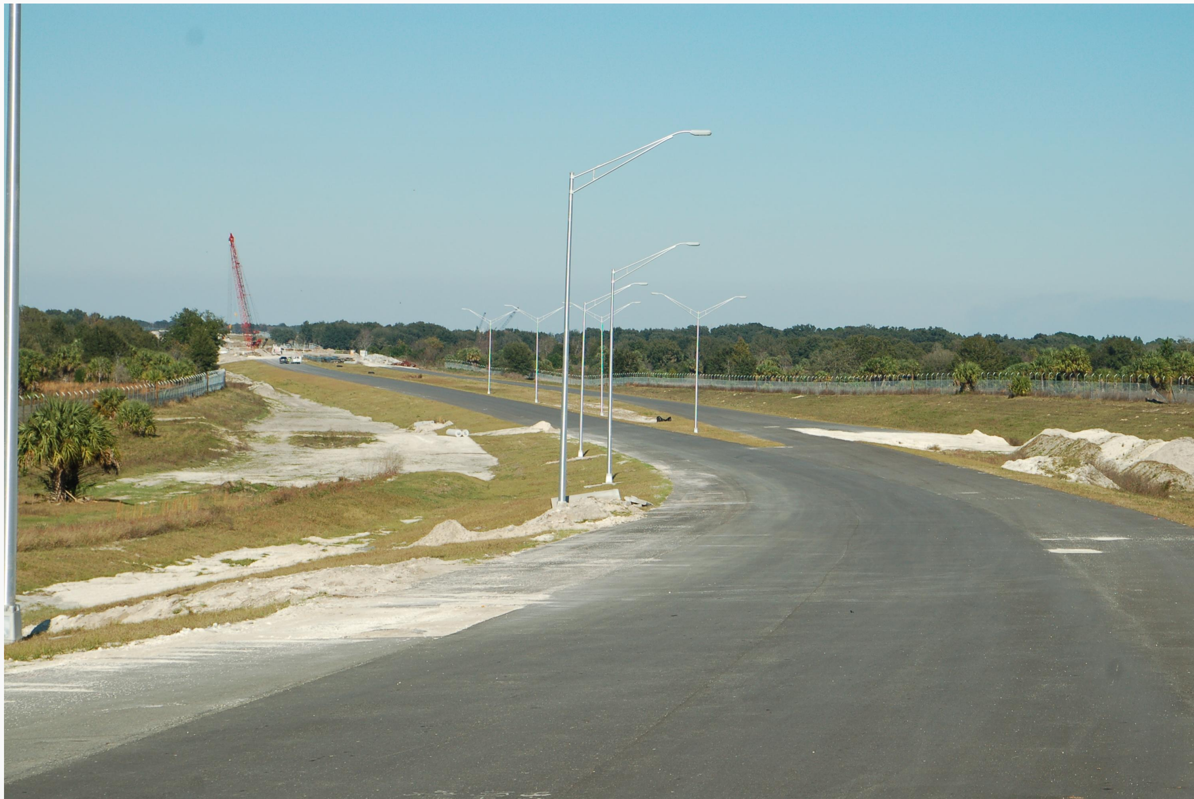
Pavement, street lights and wildlife fencing on Section 4A near CR 435 (Mt. Plymouth Rd.)
